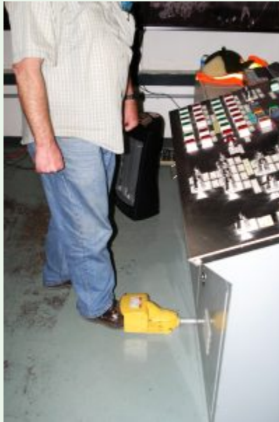
Figure 11.4: A worker must have their foot pressing the 'dead man's switch' for the control panel to operate
