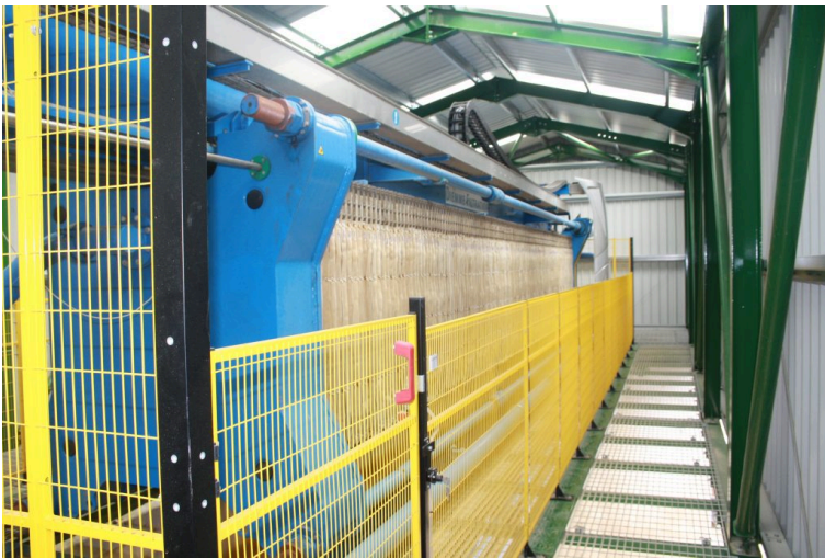
Figure 11.2: Moving parts of a machine are guarded by a yellow safety fence
