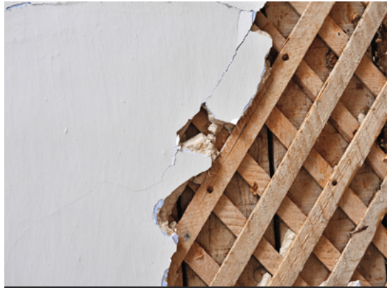
Fig.05/11 Plaster application over cross wood lath can still be found in some older housing.
