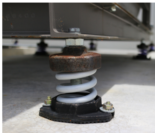
Fig.03/24 Resilient pads and coils are used to minimize transfer of equipment vibrations to the building.
