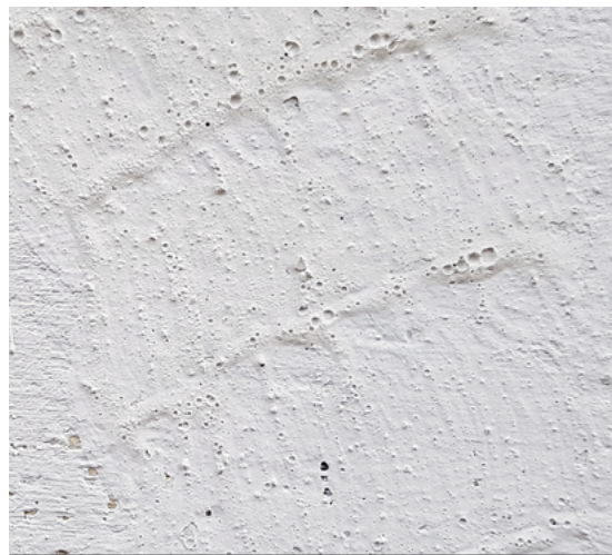
Fig.05/03 In order to mitigate the tiny craters, defoaming agents should be mixed in the paint formula.
