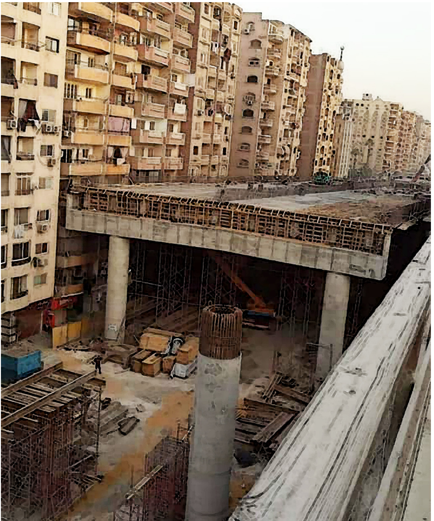
Figure 1: Where urban transport systems and residential functions meet. The picture shows the construction of the Teraet Al-Zomor Bridge in Cairo. Its edges are within arm's reach of people's balconies and it overshadows at least four storeys. Image credit: Mostnir Shady Ahmed (2020), https://www.facebook.com/mostnir/posts/10221856461623192 (Accessed on 26 Feb 2021). Printed with permission.
