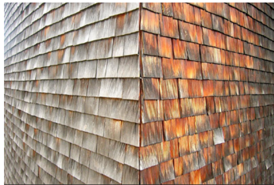
Fig.07/09 Wood shingles on different facades clearly depict the weathering effect of UV exposure.
