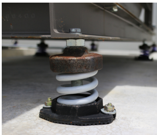
Fig.03/24 Resilient pads and coils are used to minimize transfer of equipment vibrations to the building.
