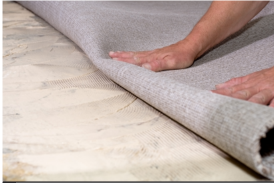
Fig.09/33 Glue-down application involves a thin layer of adhesive on a smooth substrate.
