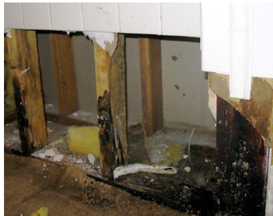
Fig.01/13 Water can easily cause destruction behind wall finishes, without the occupants ever noticing.
