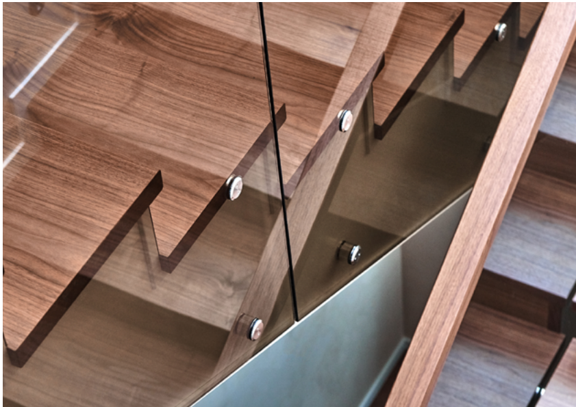
Fig.12/11 Complex details with low tolerance require impeccable workmanship, often stressing project schedule and budget.
