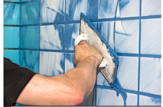
Fig.08/25 Without the use of grout release, colored grout applications can easily stain white tiles.
