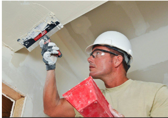
Fig.05/15 Skim coating involves a continuous layer of joint compound over finished drywall application.
