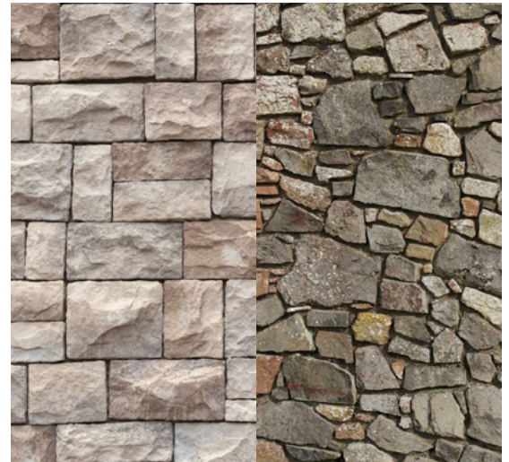
Fig.06/24 Ashlar masonry (left) is a stark visual contrast against rubble masonry (right).
