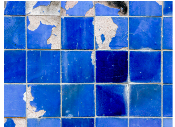
Fig.08/20 The layer of glaze on ceramic tiles is actually thin, can crackle and wear off over time.
