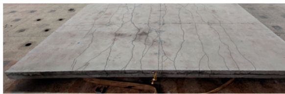
(a) Crack distribution at slab bottom
