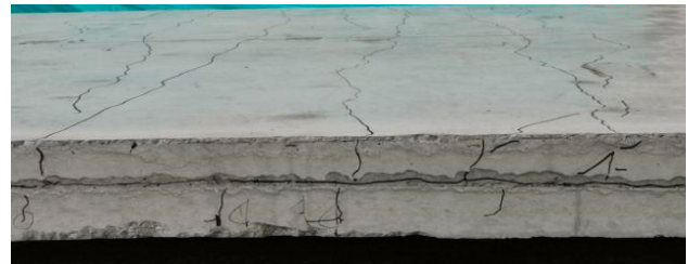
(b) Crack distribution at slab bottom
