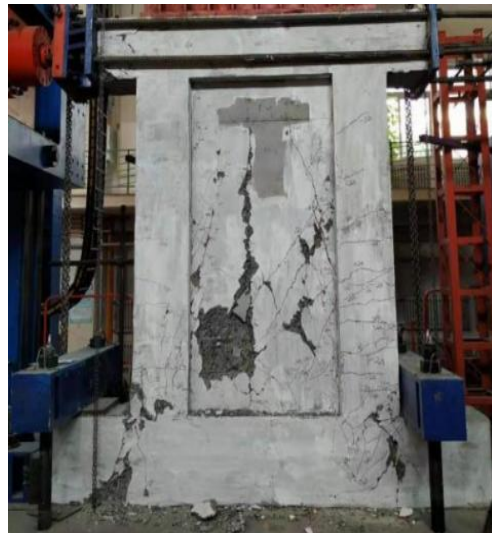
Figure 7. Final damage of specimen XJ.
