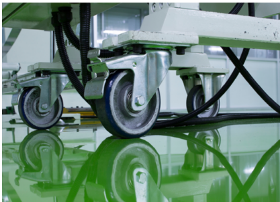
Fig.11/21 Epoxy flooring is actually a thin resin layer and requires meticulous substrate preparation.
