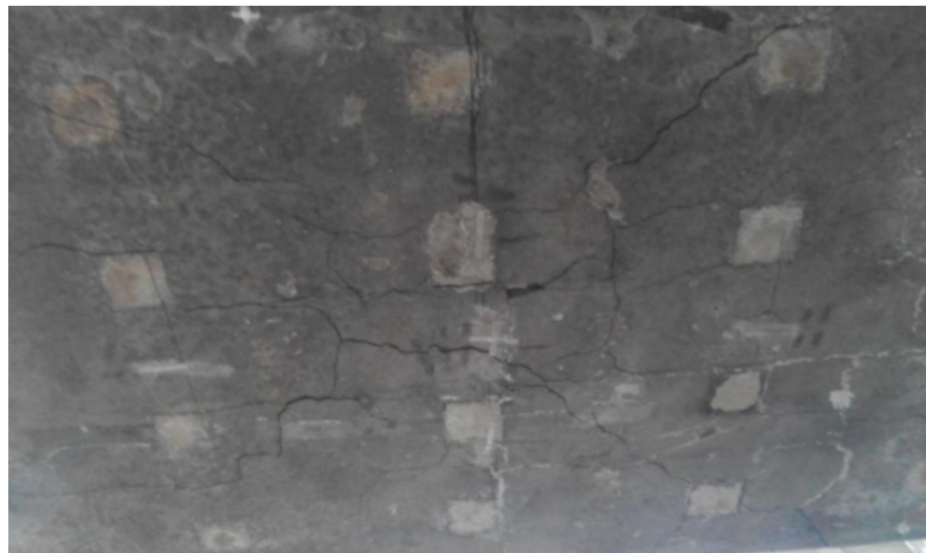
Figure 13. Failure of the precast bottom slab.
