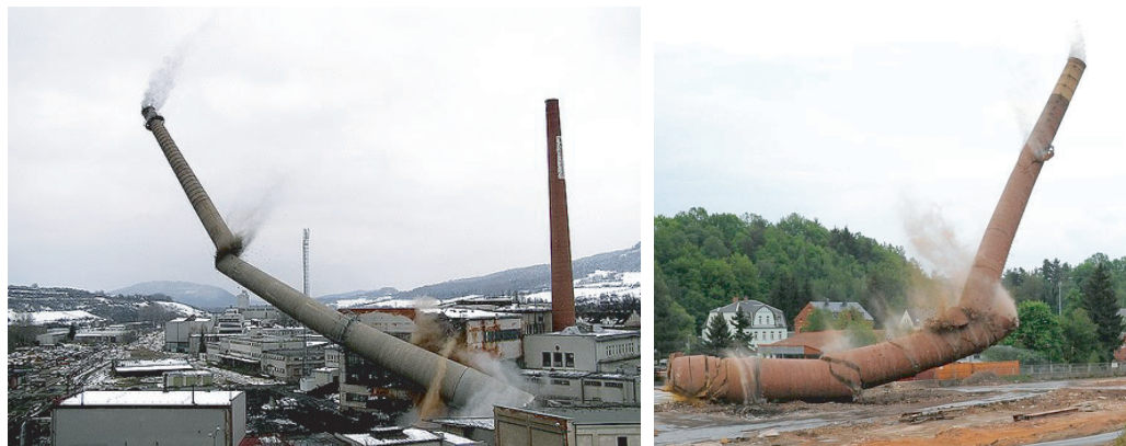
FIGURE 325 Falling brick chimneys – thus with limited stiffness – fall with a V shape (© John Glaser, Frank Siebner).
