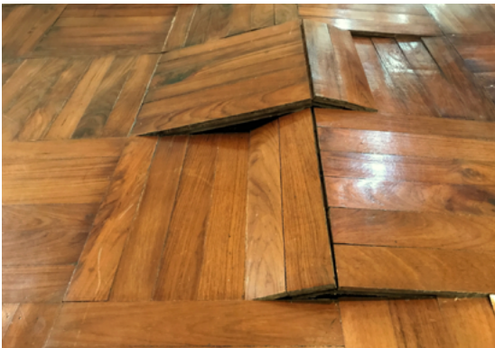
Fig.07/29 Moisture content of the environment causes the wood to expand and contract.
