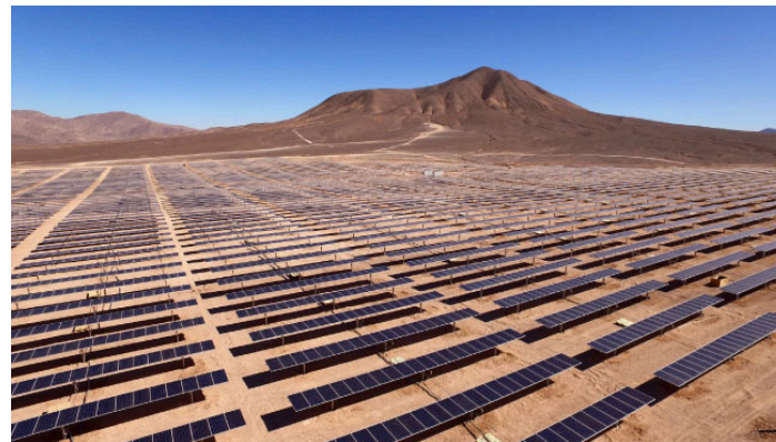
FIGURE 7.28 Solar cell arrays at a power plant in California (credit: Bureau of Land Management, Flickr)
