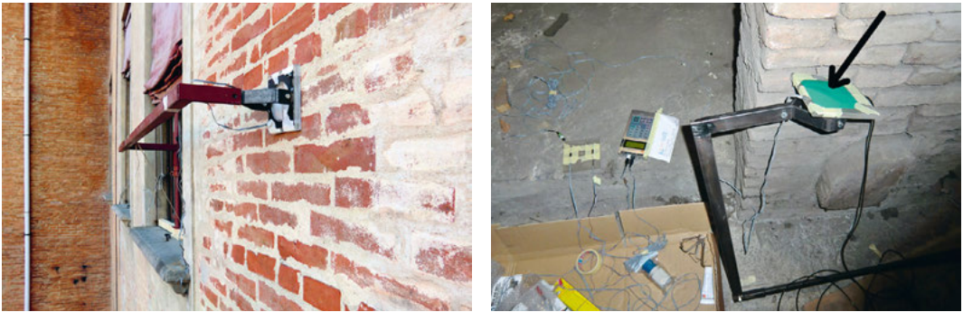
Fig. 3.18: Steel bracket to hold sensors in place and thermo-conductive foil pad for U-value measurement
