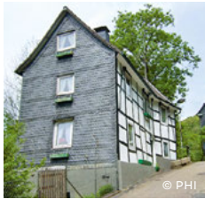
Fig. 2.8: Slates as protection against driving rain on the windward side of a traditional German half-timbered house
