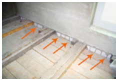
Fig. 5.9: Absence of interior plaster in the depth of the wooden beam ceiling, exposed during modernisation work
