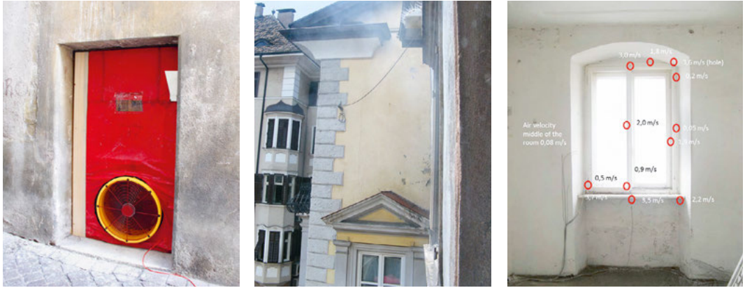
Fig. 1.9: Fan installed in the entrance door; gas overflow through window; measurement of air velocity at a pressure difference of 50 Pa at several points of the existing window. The blower door test for the building resulted in nearly 10 1/h, value
