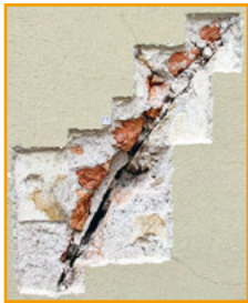
Fig. 3.10: Masonry arch documented by IRT and break opening as part of the construction history of the Waaghaus
