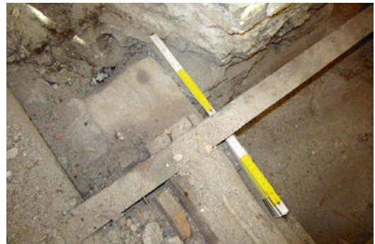
Fig. 1.7: Several wooden beam-ends in the ceilings of the 1st and 2nd floor were exposed to visually diagnose their exact position, how they bear on the exterior wall, and what their condition is.
