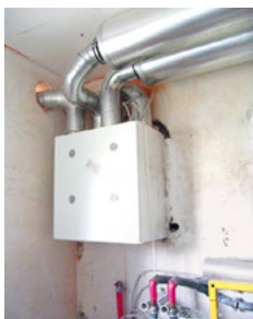
Fig. 2.7: Installation of a heat recovery ventilation system in a retrofitted building. The white box is the ventilation unit with fans, filters and the heat exchanger. Visible at the top right are sound absorbers that eliminate any fan noise.
