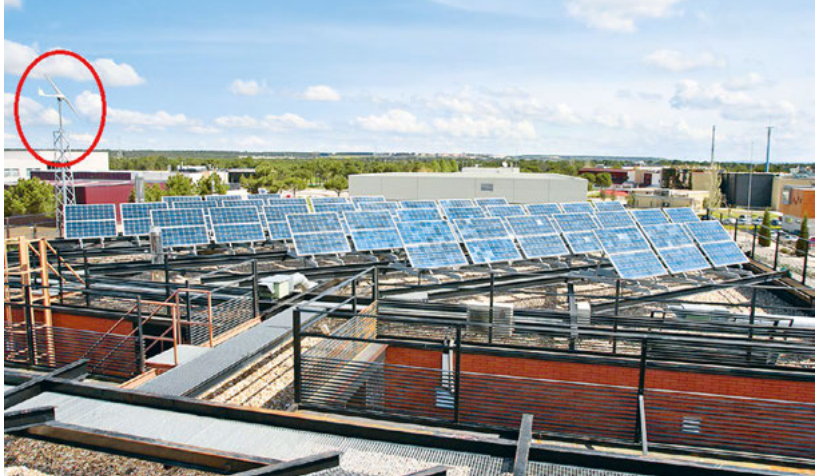
Fig. 5.70: Wind turbine fixed to a building
